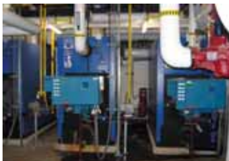
A much-needed boiler upgrade revealed other problems.
