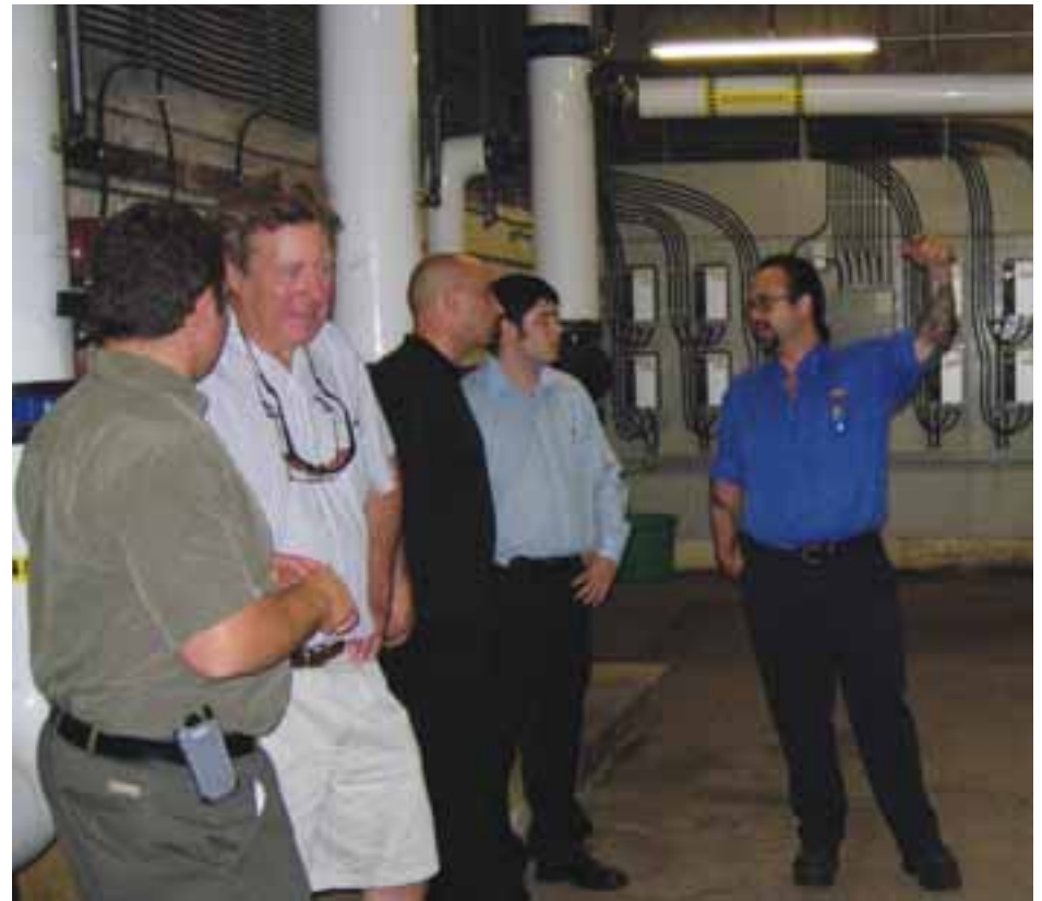
From left, mechanical contractor Dave De Faveri, engineer Fred Weinstein, filter supplier John Priolo, Nick Campbell of Allied Technical Services and building superintendent Paul Nelson discuss the project.
