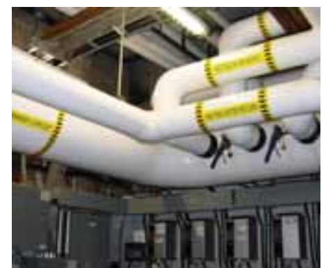
Pipe fitting as fine art – note the variable speed pump drives below.
