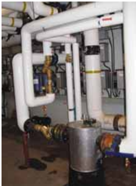
This European-made magnetic sludge separator provided a cure.
